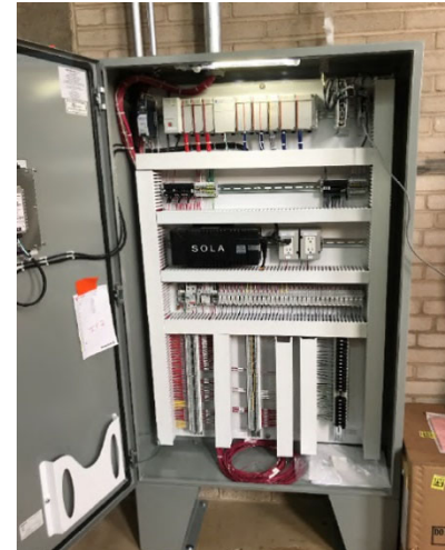
Main Control Panel
