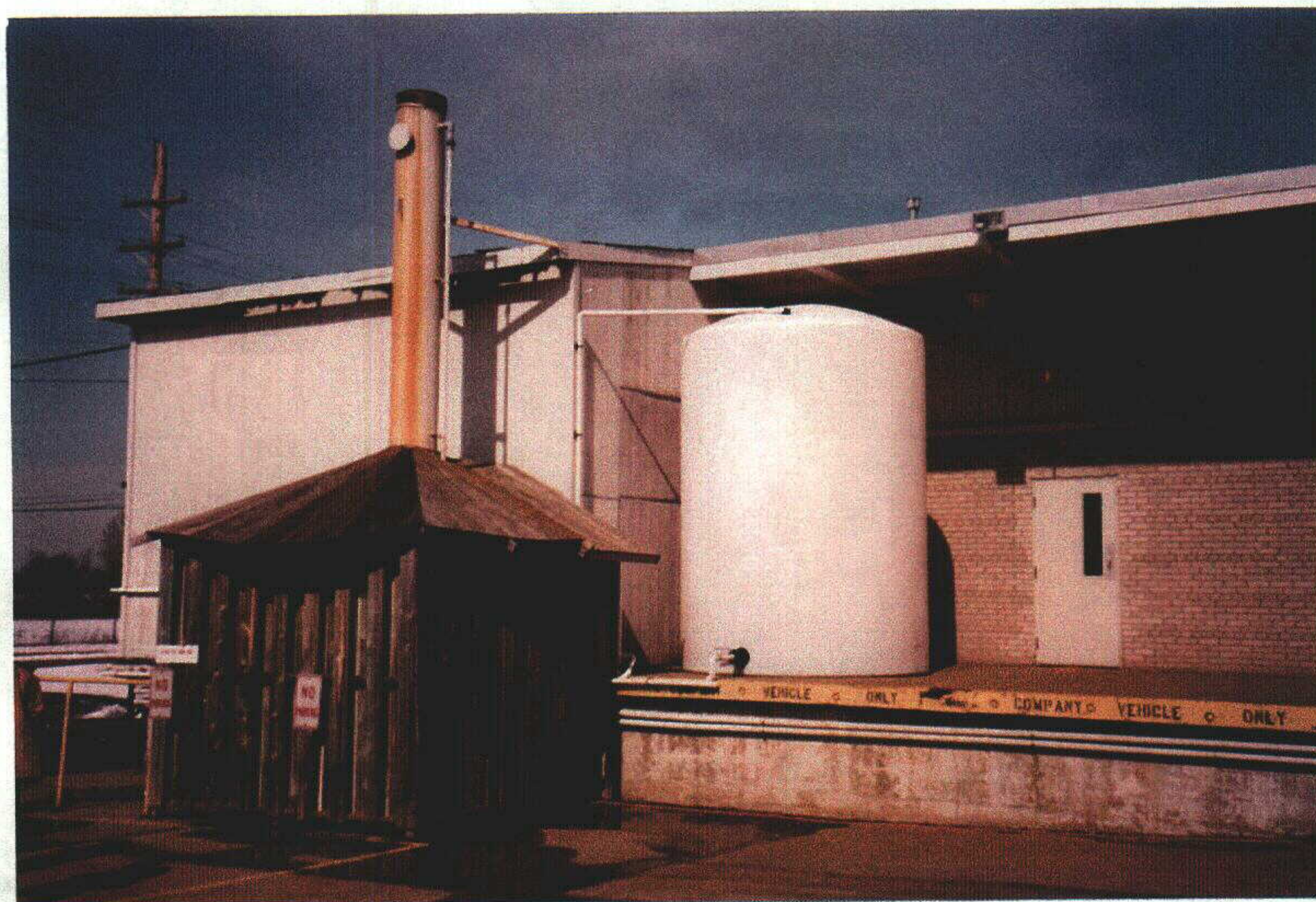
Photograph #6: Site A Groundwater Treatment System (OU2)
