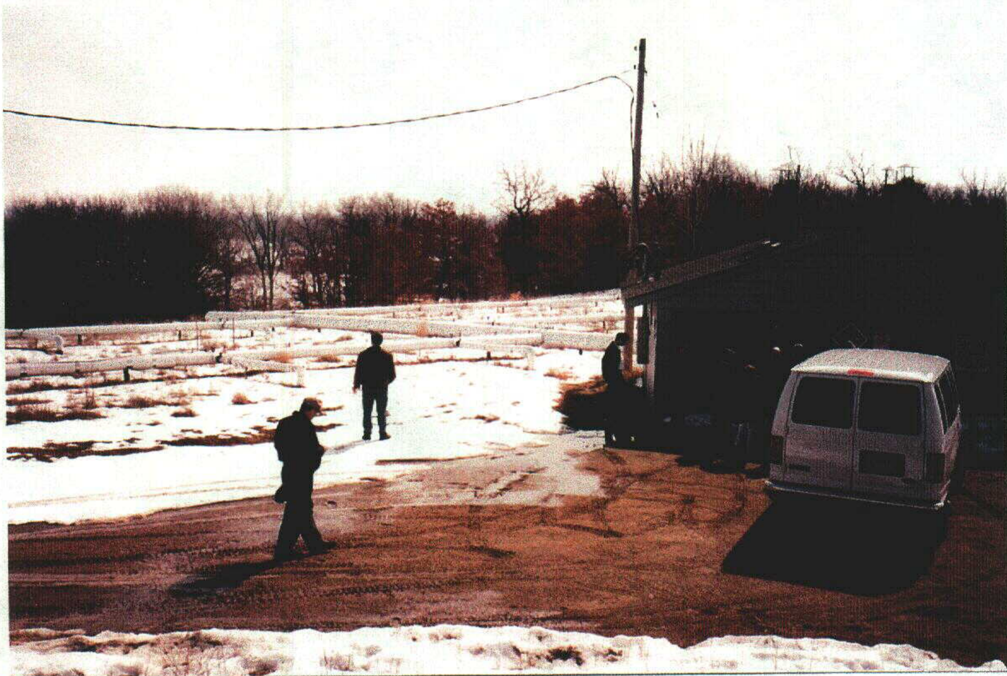
Photograph #5: Site D Shallow Soil SVE System (OU2)
