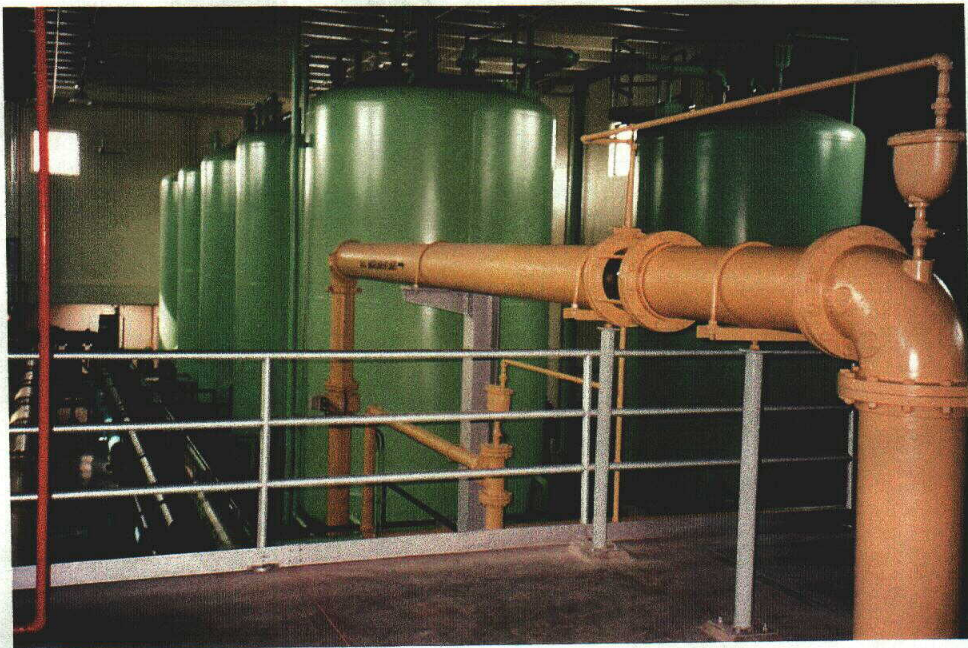
Photograph #7: PGRS Water Treatment Facility (OU3)
