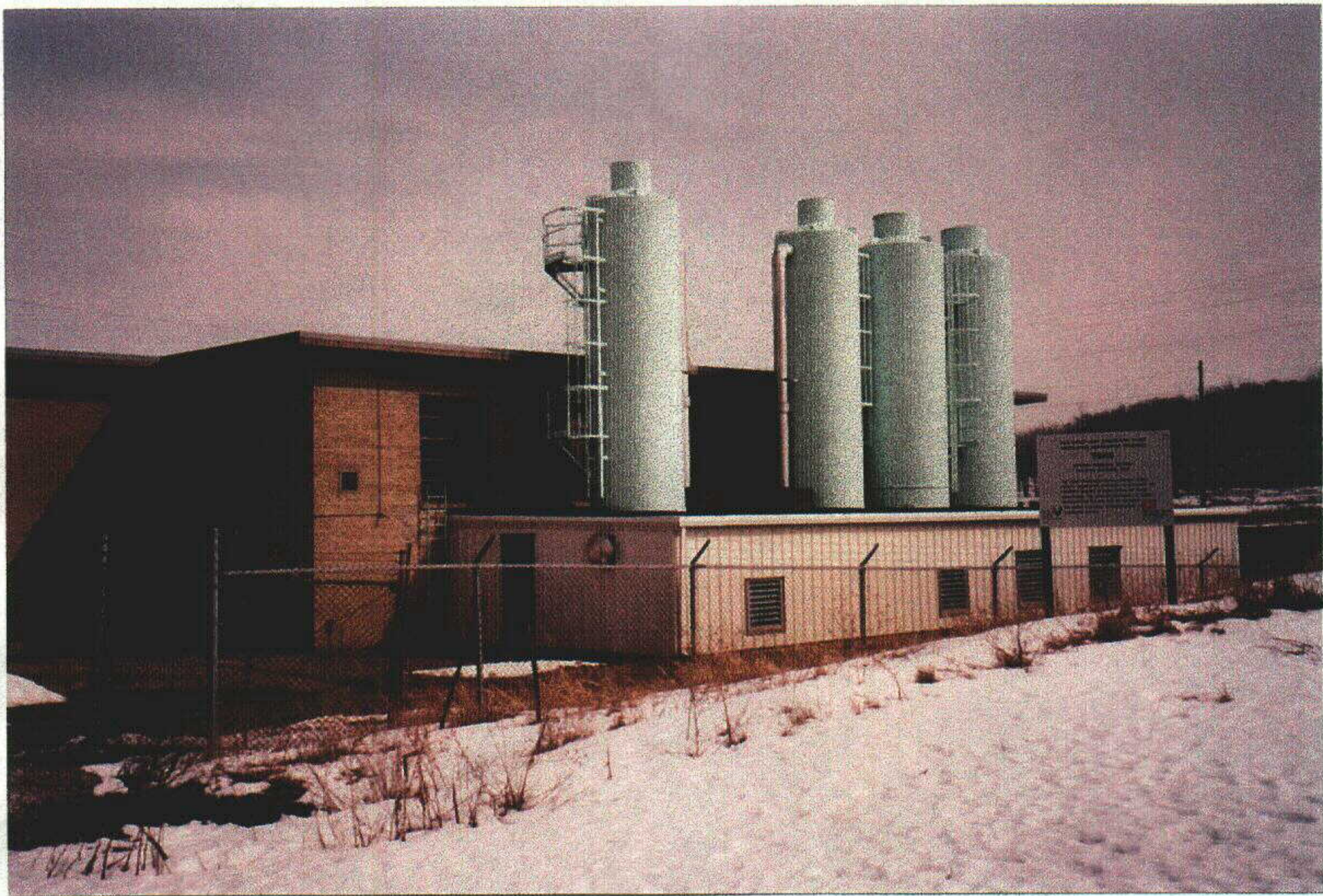
Photograph #3: TGRS Water Treatment Plant (OU2)
