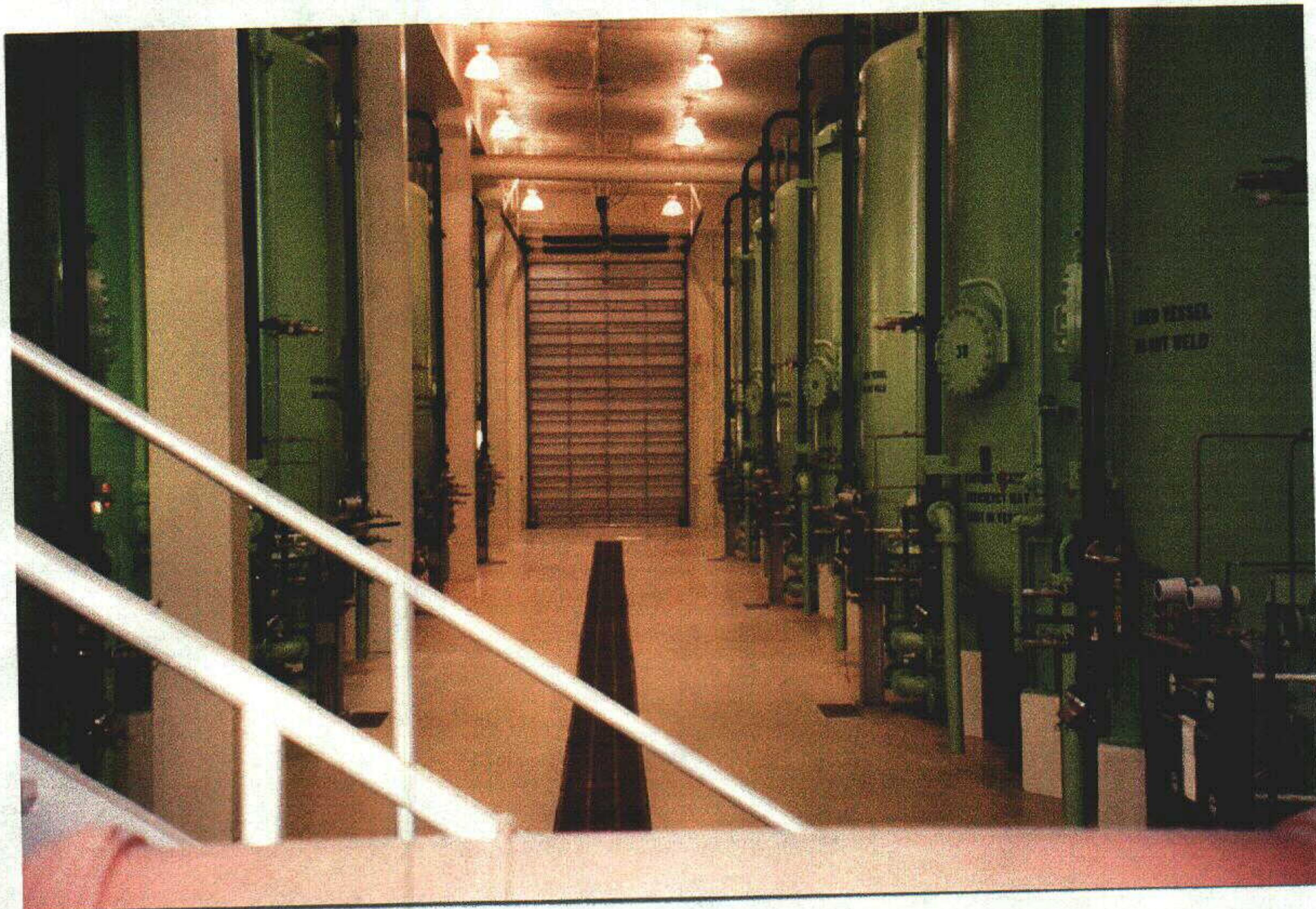
Photograph #1: PGAC Water Treatment Facility (OU1)
